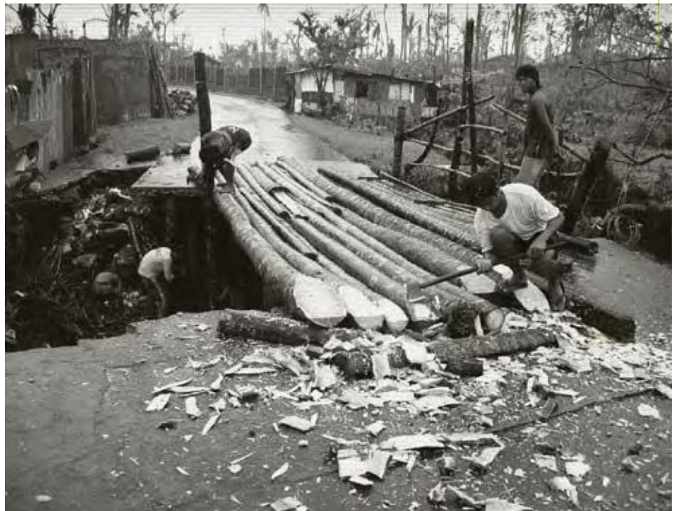
Repair costs should be considered when measuring the impact of climate change. Residents of Barangay Santa Teresa in the municipality of Malillipot, Albay, in the Philippines, repair their bridge following a typhoon in 2007. Photo: Maria Socorro Melic/World Vision
